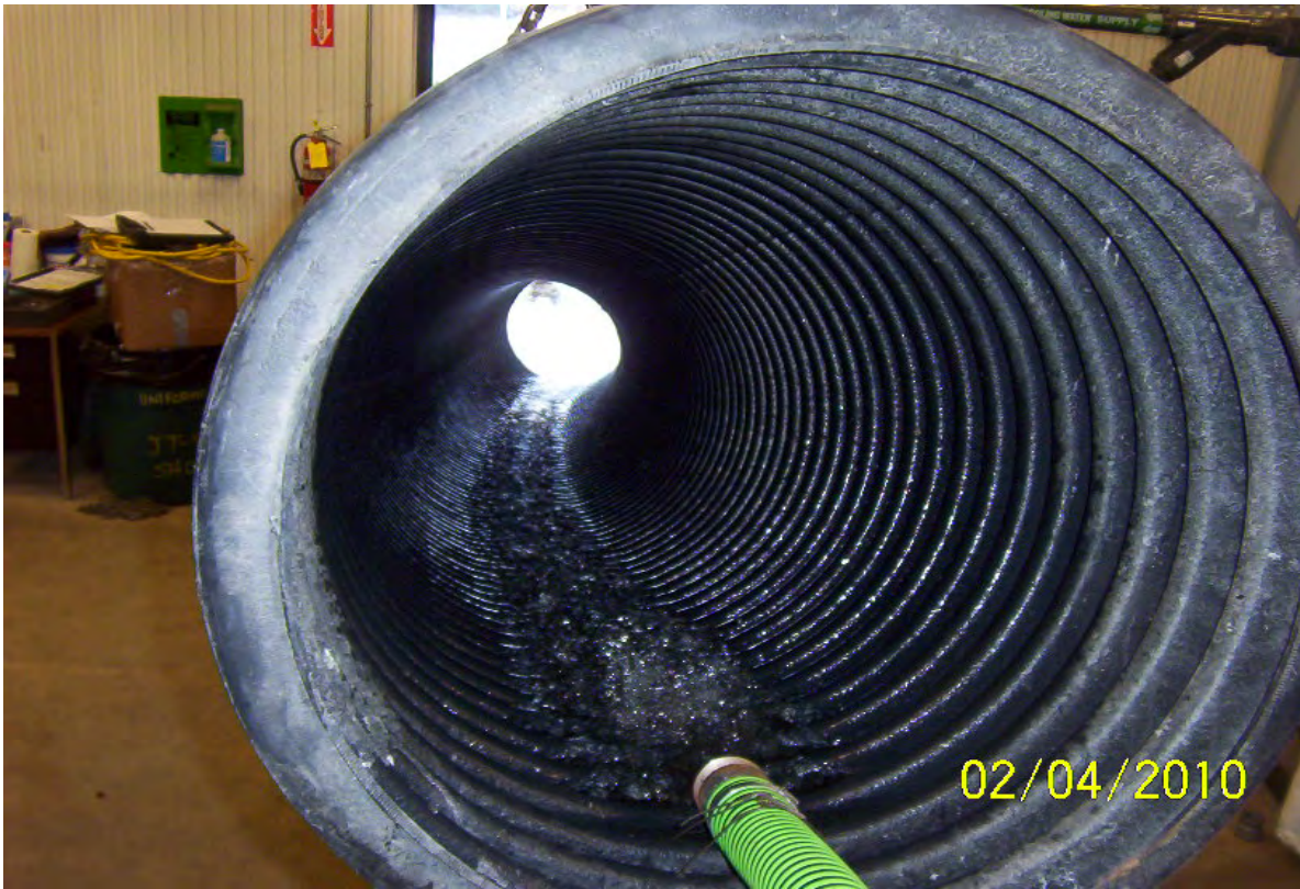
Photo 1: Typical Pipe Flow, approx. 50 gpm, 24 inch HDPE corrugated pipe
